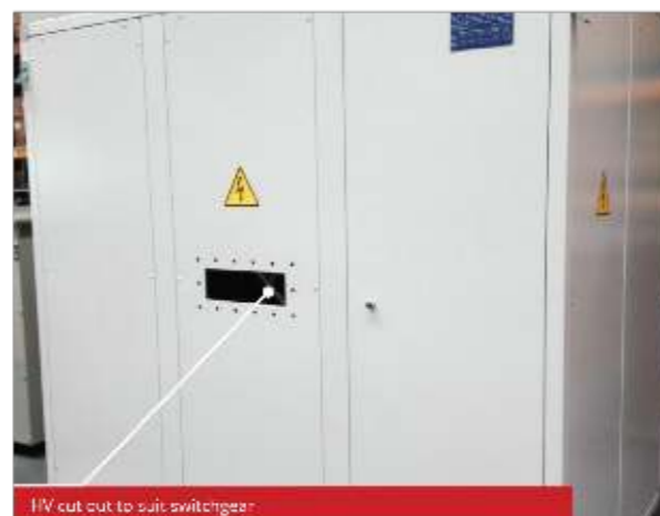
HV cut out to suit switchgear
