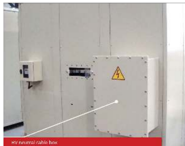
HV neutral cable box
