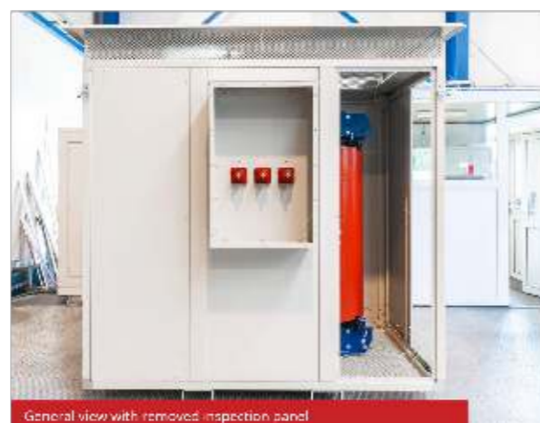
General view with removed inspection panel
