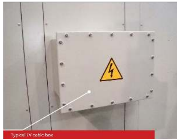
Typical LV cable box
